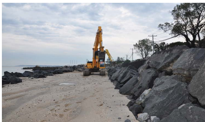
As part of the rehabilitation project a Corps of Engineers contractor places 5 to 7 ton boulders as part of the breakwater. Photo Credit: Dan Desmet, Public Affairs
